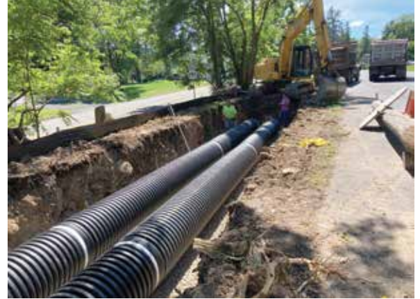
An underground stormwater infiltration trench along Route 390 near Mountainhome United Methodist Church. The trench allows rainwater to filter slowly into the ground without rushing into nearby creeks.
