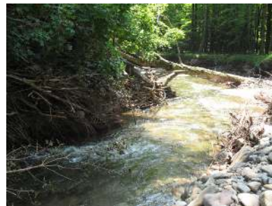
Fig. 4 Serious bank erosion site
