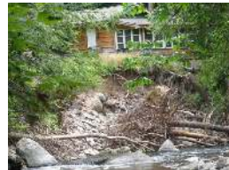
Fig. 2 Serious cutting of the stream bank
